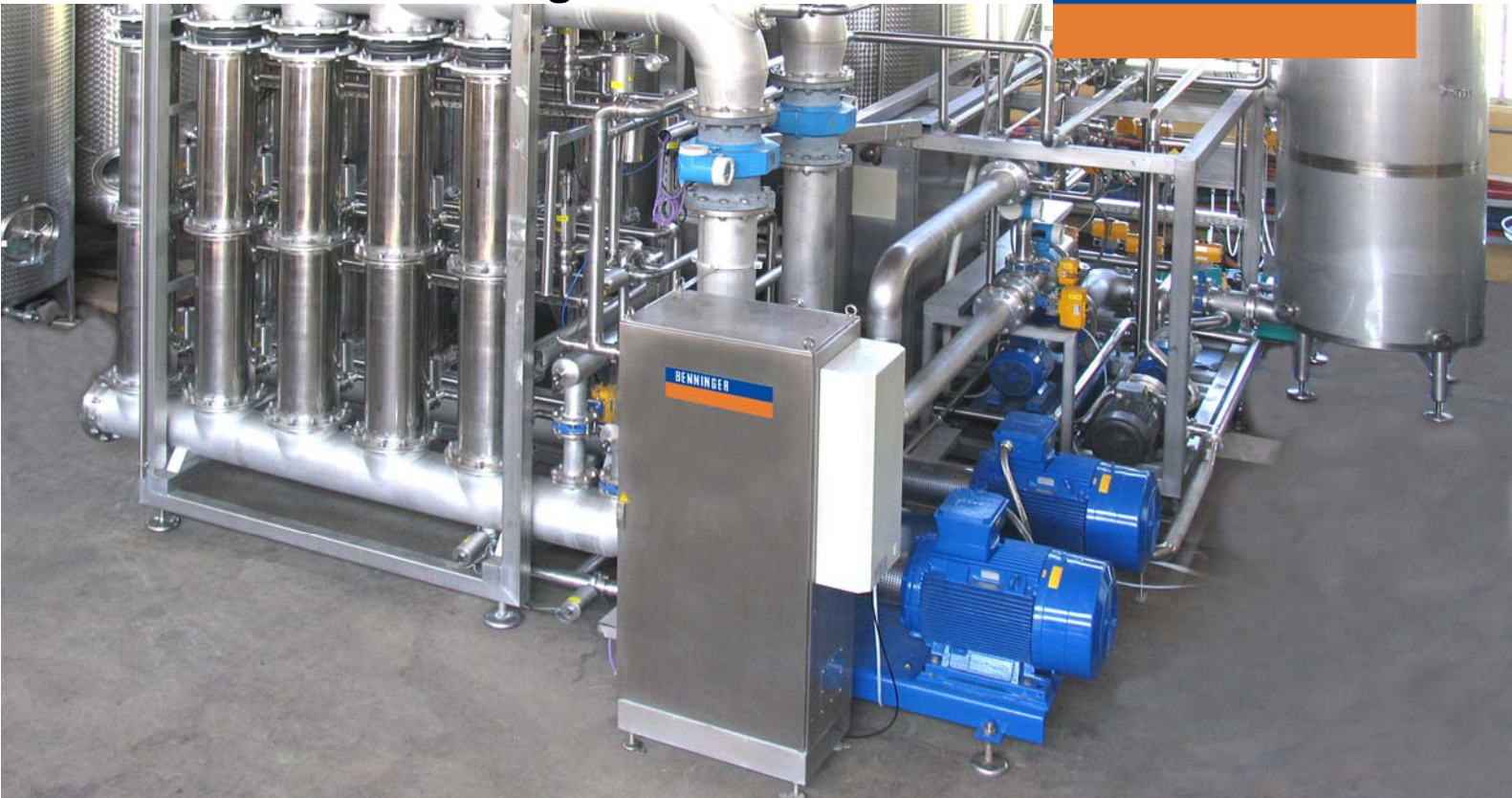
UF system for approx. 20 m 3 /h
